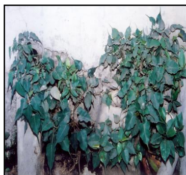
Fig.11. Ficus religiosa L. (Pipal) growing from a leaking and damaged sewage line of Islamia College building.
