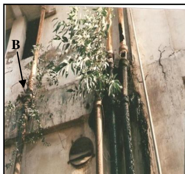
Fig.10. A. Eucalyptus citriodora Hook left and B. Salvadora persica L. (Peelu) right, growing from the damaged leaking sewage pipe of a Govt. office building, Gulshan-e-Iqbal.
