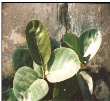
Fig.7. Ficus bengalensis L. (Burgad) growing near leaking sewage line. Islamia College building.
