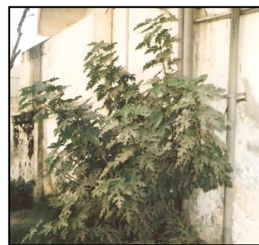
Fig.12. Ficus johannis Boiss growing from the damaged sewage line of a residential building.
