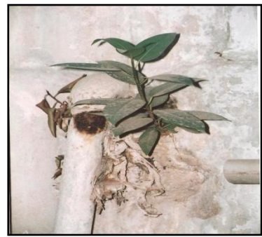
Fig.3. Ficus rumphii Blume is propping from the crevices of the Adamjee G.S.C. building near the damaged sewage line.
