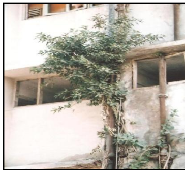
Fig.2. Ficus rumphii Blume growing from a crack of the Adamjee Govt. Sci. College caused by a leaking sewage pipe.
